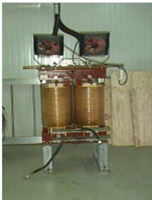
Short-circuit test up to 42kA/2Sec
